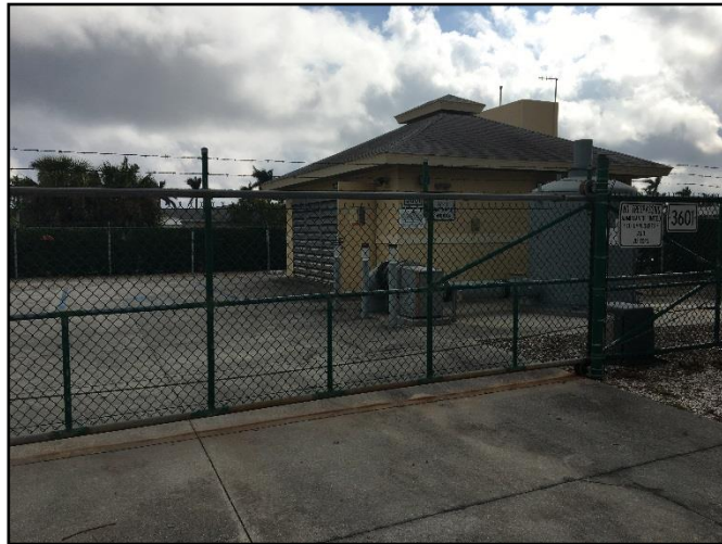
Figure 11: Lift Station - Cape Coral
