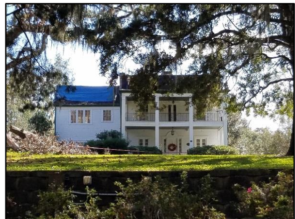
Figure 16: Leu House with structural damage from Hurricane Irma
