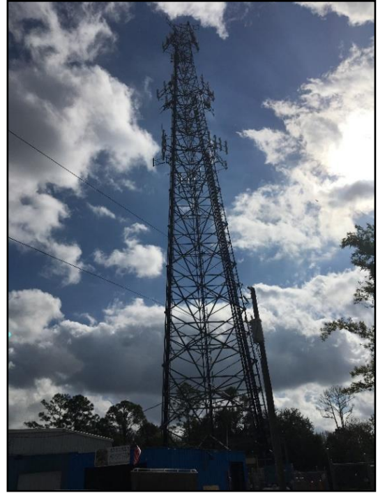
Figure 9: Cell Tower in Charlotte County
