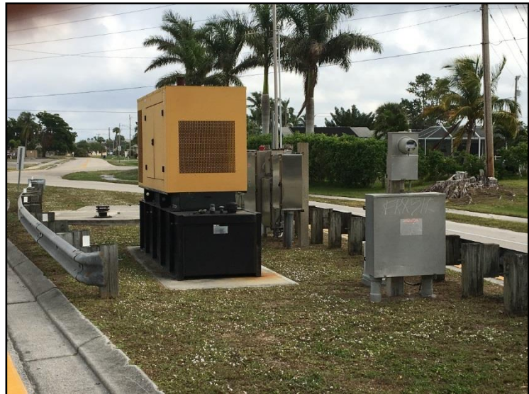
Figure 12: Back up Emergency Power for a Lift Station-Cape Coral
